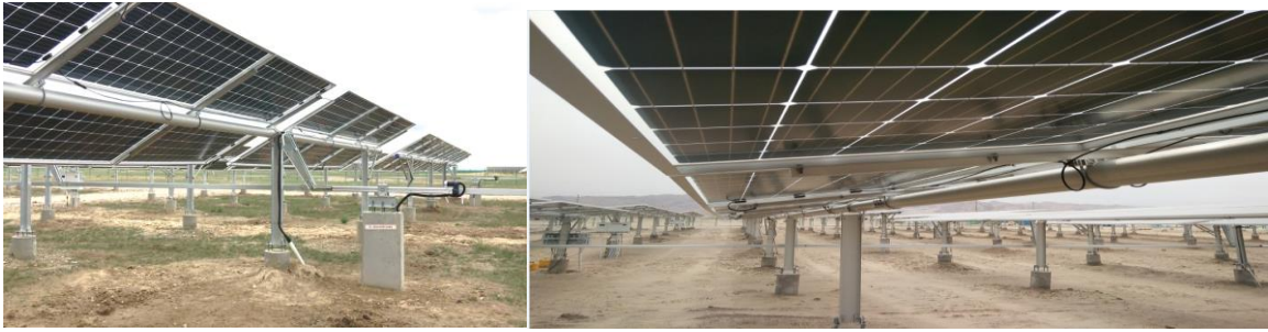
5.5MW bifacial modules project in Qinghai, China
